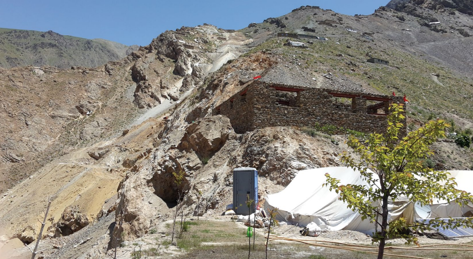
Fig. 4: A new house being constructed near an emerald mine shaft using host rock from the mine. Outside the home is a toilet which is a new concept in this mining area. (Photo by Shahiq Habibi)
