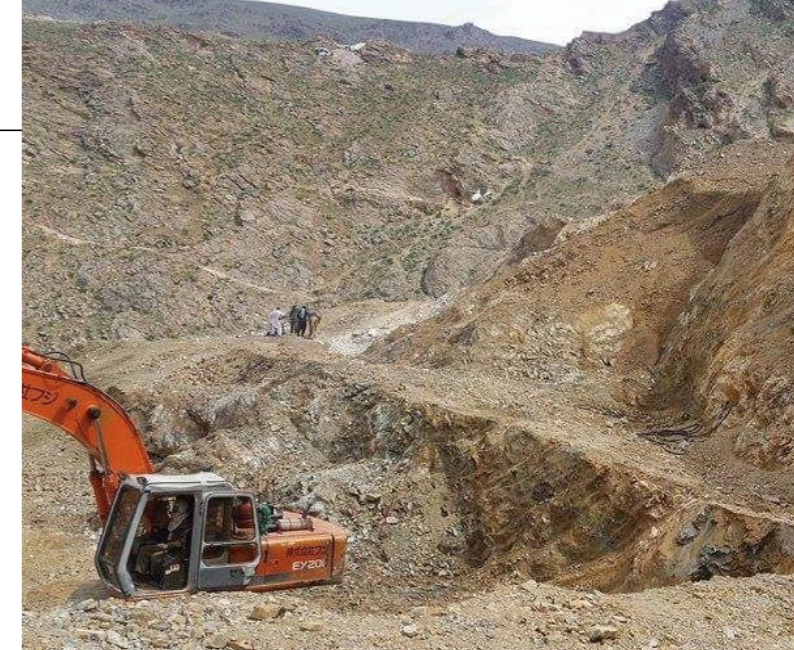
Fig 20: Heavy equipment is being used to rapidly remove overburden at the mine site. It will be interesting to see what emeralds are discovered as the open pits are deepened. (Photo by Shahiq Habibi)
