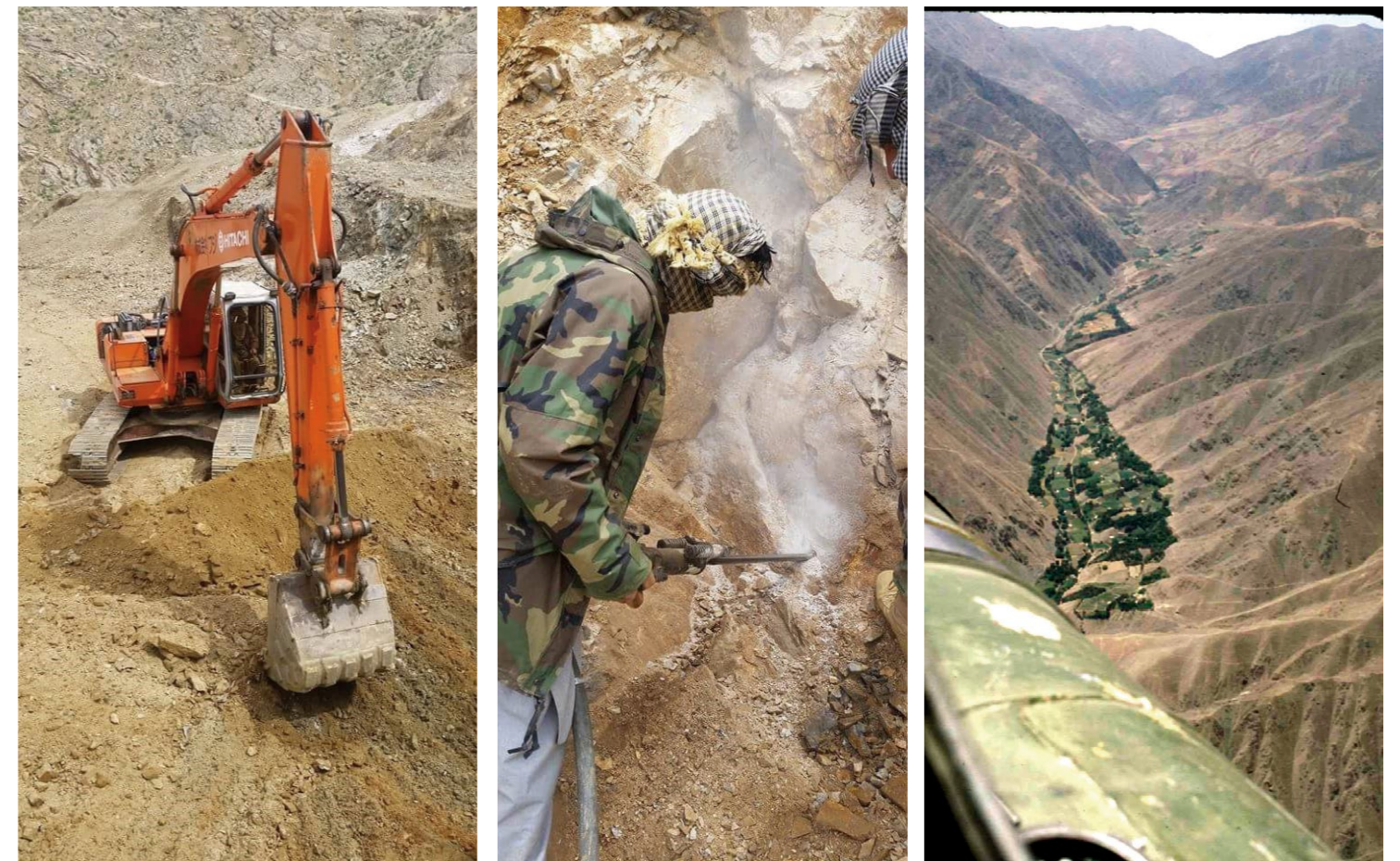
Fig. 15 (left): Heavy equipment is now being used in the emerald mining operations. (Photo by Shahiq Habibi)
