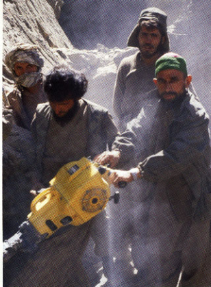
Figure 8. Diesel-powered drills are also used to remove the hard wallrock. Because the miners wear virtually no protective gear, injuries from falling or flying rock—as well as illness from the carbon monoxide fumes—are common. Photo by Gary Bowersox.
